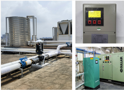
Efficient energy generation: Huizhou plant utilises waste heat from air compressors and photovoltaics to reduce emissions
