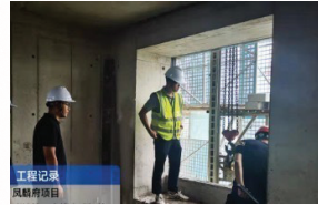
On-site safety inspections and safety disclosure training 現場安全巡查暨安全交底培訓
