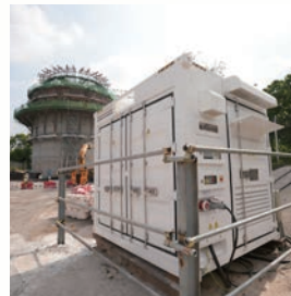
Battery energy storage system (BESS)
