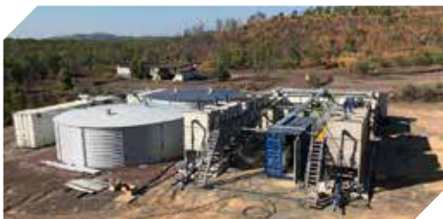
Wastewater Treatment Plant
