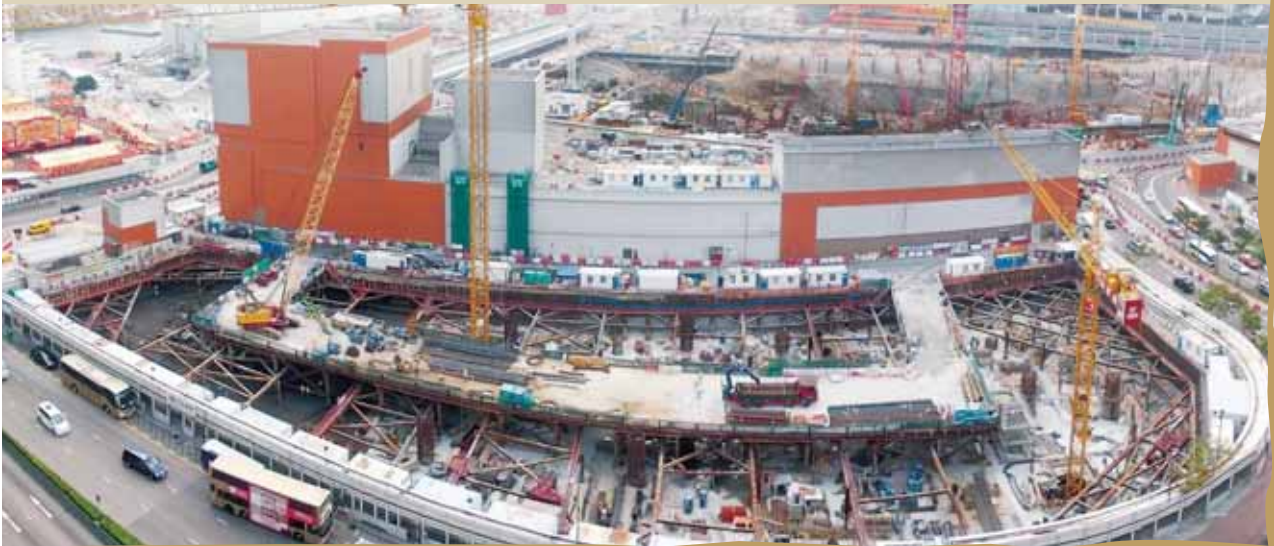
Main Contract Works for Proposed Residential Development at Austin Station Site D at K.I.L. No.11129, Kowloon
