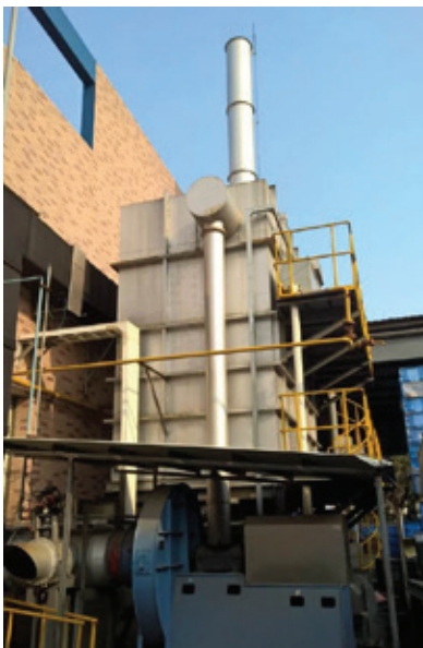
RTO waste gas treatment facilities
