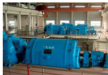
Steam Turbine Generator
