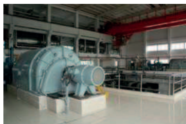
Steam Turbine Generators
