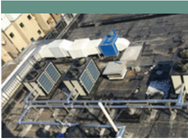
Air source heat pump
