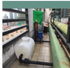
Cooling water tower
